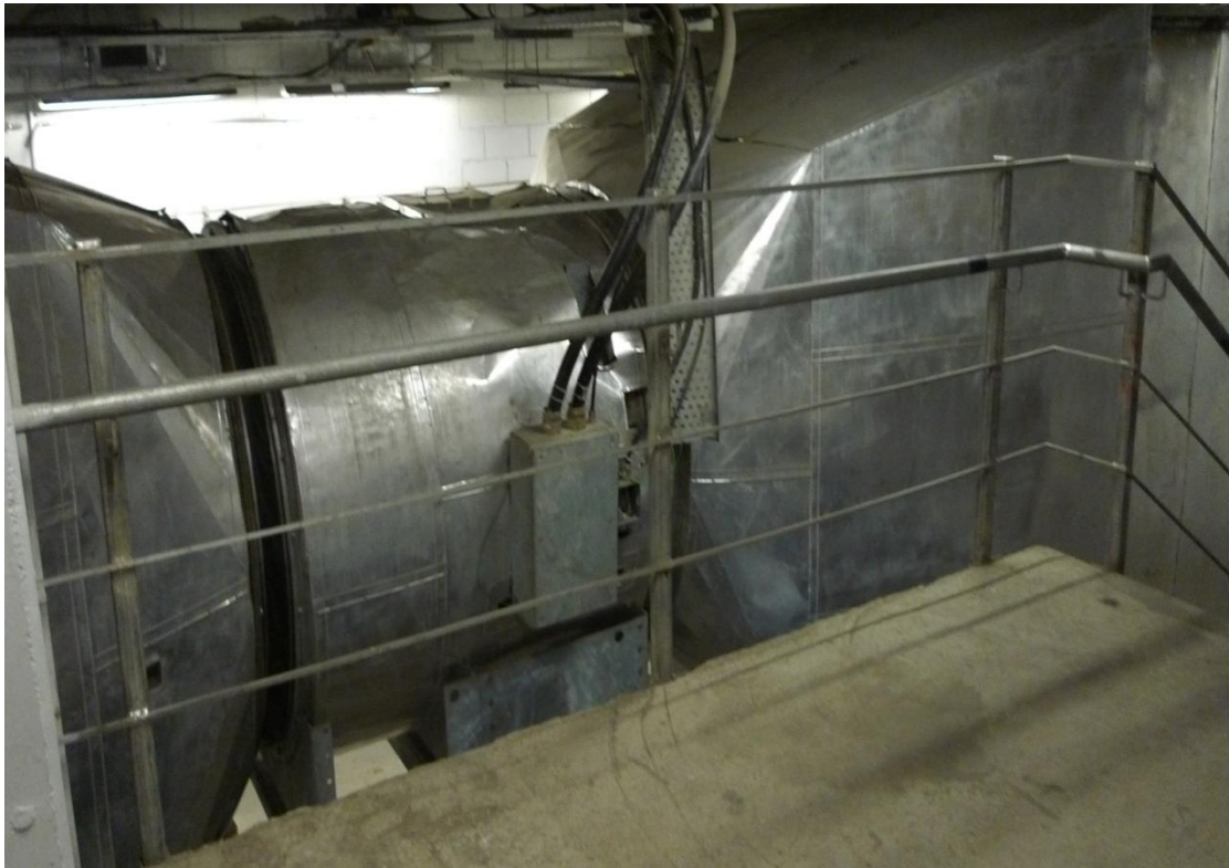
Figure 9-2: Trackway Exhaust Fan
