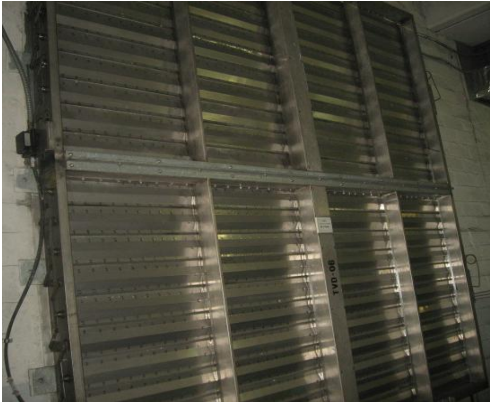
Figure 9-1: Tunnel Ventilation Dampers
