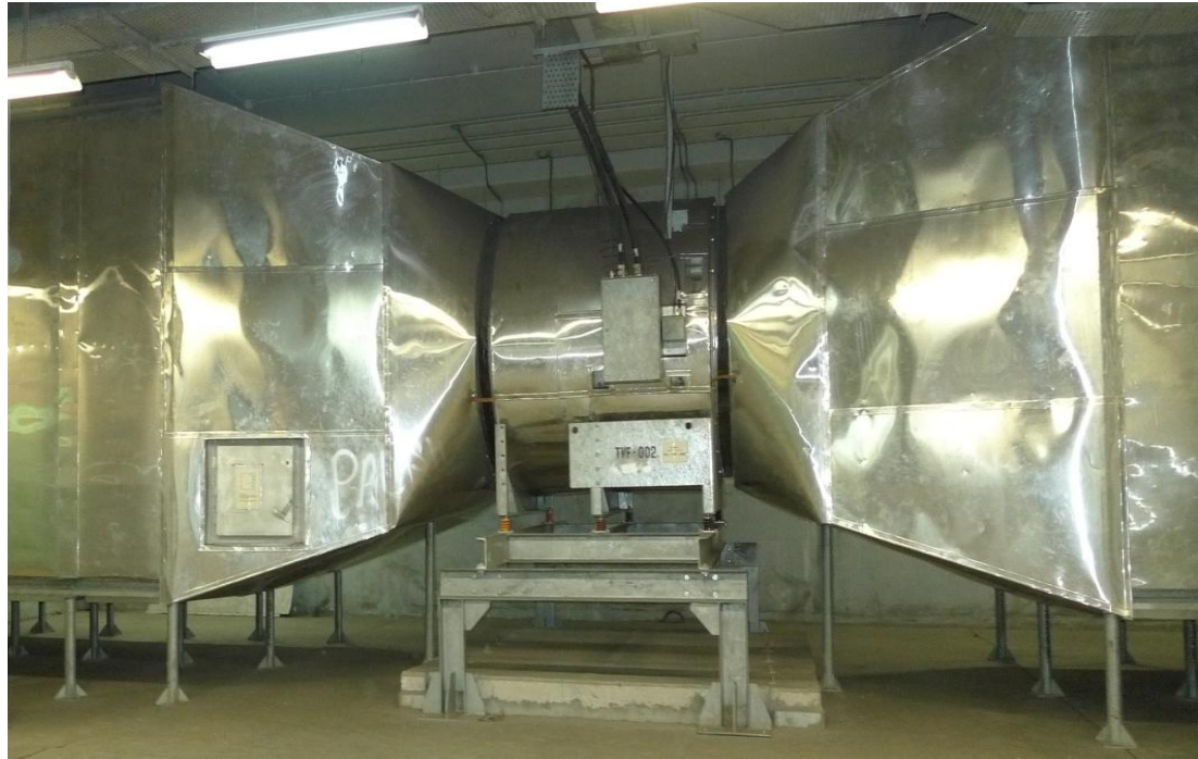
Figure 9-3: Tunnel Ventilation Fan
