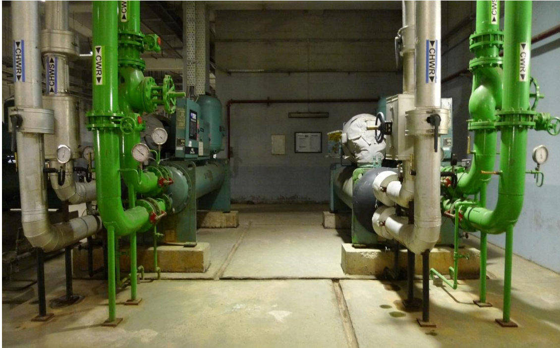
Figure 9-5: Chiller Plant Room
