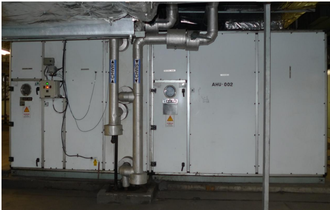
Figure 9-4: Air Handling Unit
